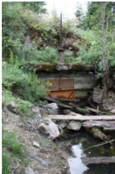
The valve works just south of Loon Lake that controlled the flow of water into the Arcadia Orchard irrigation system.
